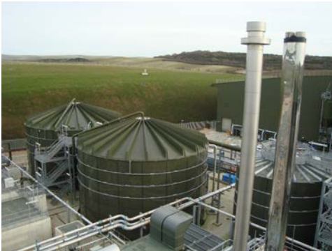
Picture 1: The newly completed works can treat the 95 million litres of wastewater generated each day by the residents of Peacehaven, Telscombe Cliffs, Ovingdean, Rottingdean, Saltdean and Brighton and Hove.
